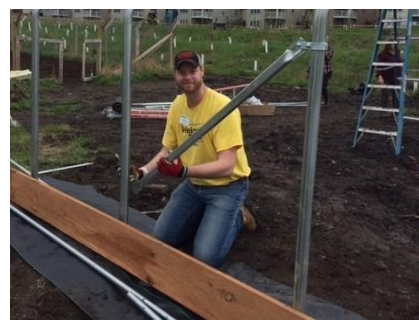
Nick Krueger volunteered to help a local charity assemble and raise steel trusses that will be wrapped with heavy gauge plastic sheeting. The completed structure, owned by Urban Roots, will grow produce to be sold locally.
