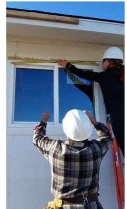
Agents at Weichert, Realtors® - Barton Harris & Co. installed new windows at a Habitat for Humanity house in Austin.
